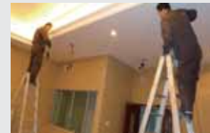
Switch circuit retrofit
