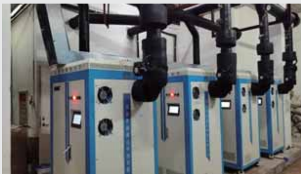
Relevant equipment for gas conversion to electricity project
