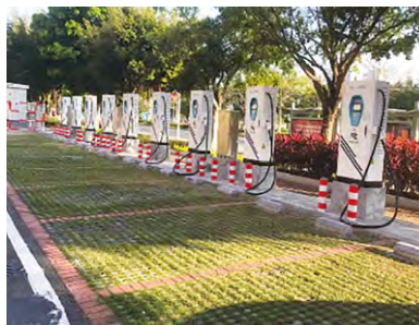
New Energy Vehicle Charging Piles
