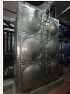
Air conditioning waste heat recovery tank
