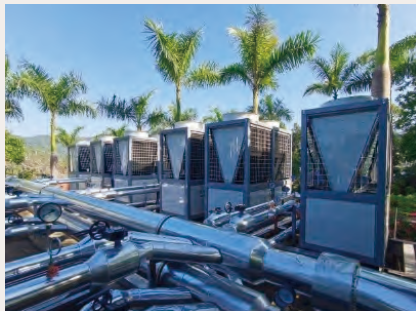
Gas to electricity equipment operation
