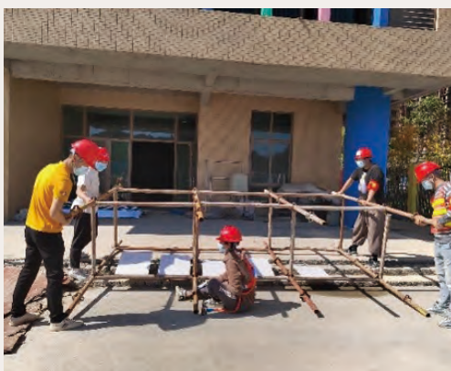
Collapsing accident drills
