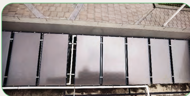
Site Solar Application
